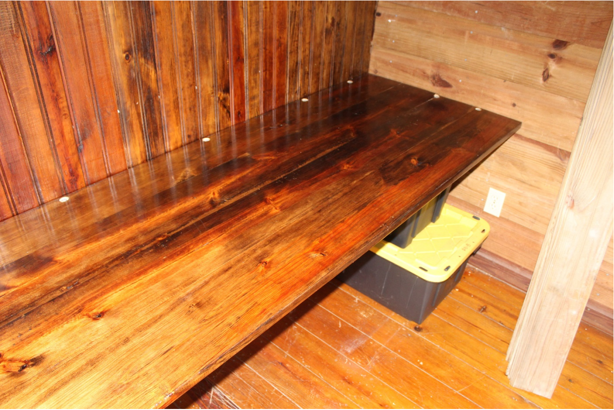
The asymmetrical location of the lag bolts is the result of them being strategically placed to correct the twisting and warp. The right-side wall will be finished in bead board to match the back wall.
