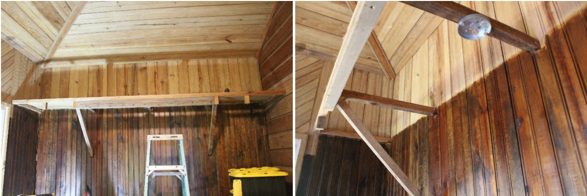
To level the canopy/shelf, would require unloading, complete disassembly and rebuilding from scratch as the bracing was not originally spaced correctly.
